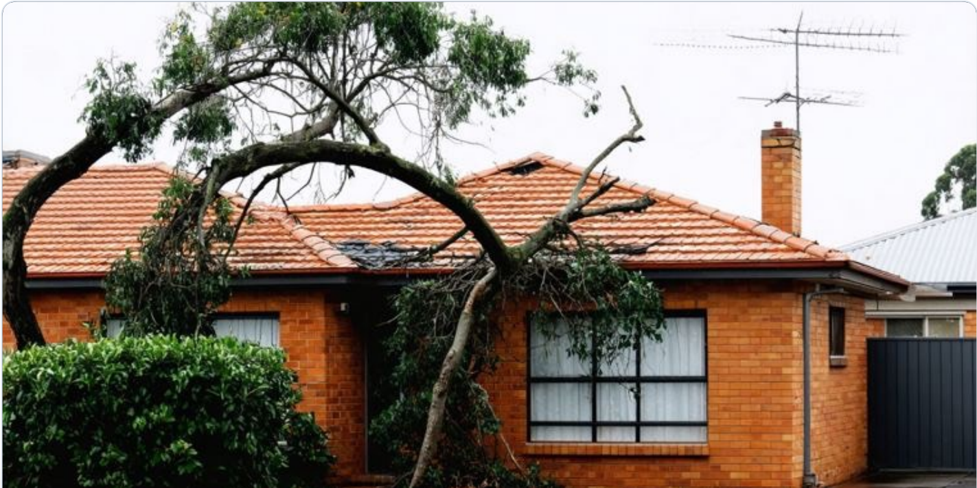
PHOTO 1 OF 3 Front of the property, tree down across the roof line
