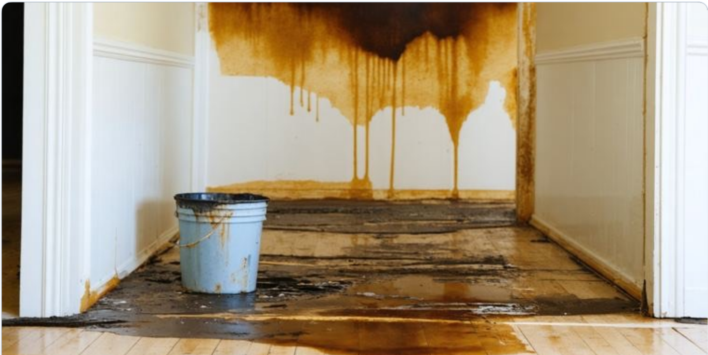
PHOTO 1 OF 3 Staining and pooling in the hallway below the ensuite
